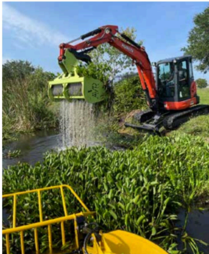
Brevard County staff uses an aquatic vegetation rake, a specialized excavator attachment designed to quickly drain water while harvesting plants. Shown here, water hyacinth—a highly invasive aquatic plant introduced into Florida in the 1880s—is being removed from a stormwater pond. Left unchecked, this aquatic plant rapidly blankets freshwater lakes and ponds, resulting in nutrient load and flooding issues. Photo: Brevard County Natural Resources Management Department
